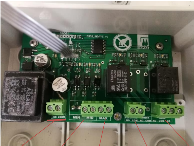
220V El. Input Bottom Floater Switch Connection Upper Floater Switch Connection Solenoid Valve 220 V Output Overflow alarm NO, COM, NC connections and electronic valve to be connected to NO and COM to empty tank incase of overflow gether with alarm Min Water level Max. Water Level To start alarm
